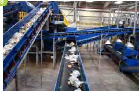
Recycling plant for industrial, business and household waste Dubai (UAE) 150,000 t/a Year of construction 2019
