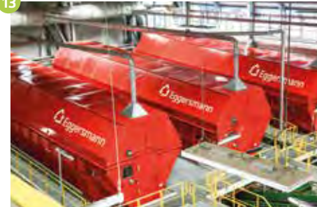
Treatment plant for business and industrial waste Tel Aviv (IL) 660,000 t/a household waste and 90,000 t/a C&I Year of construction 2015, expansion 2021
