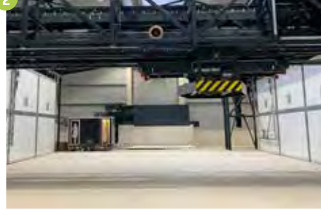
Composting plant with composting tunnel and mechanical treatment for organic waste, green waste and compost Anröchte (DE) 43,000 t/a Year of construction 2020
