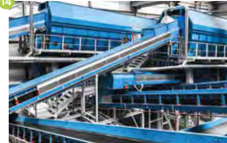
Mechanical treatment for household waste Bargeddie (UK) 190,000 t/a Year of construction 2019
