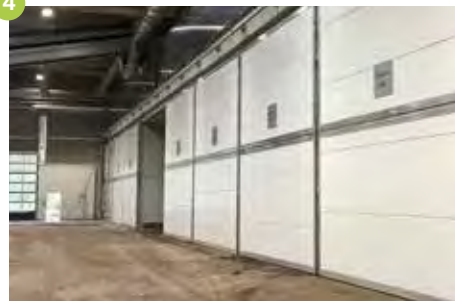
Composting plant with composting tunnel and mechanical treatment for organic waste, green waste and compost Lünen (DE) 75,000 t/a Year of construction 2019
